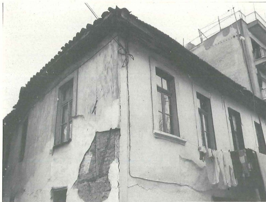
House in Kioupri; most houses in the area are in a dilapidated state
